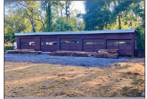
5-BAY FRAME GARAGE
