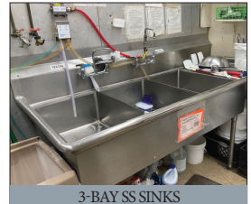
3-BAY SS SINKS
