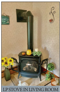
LP STOVE IN LIVING ROOM
